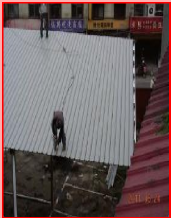
Before 屋頂作業未有防護
