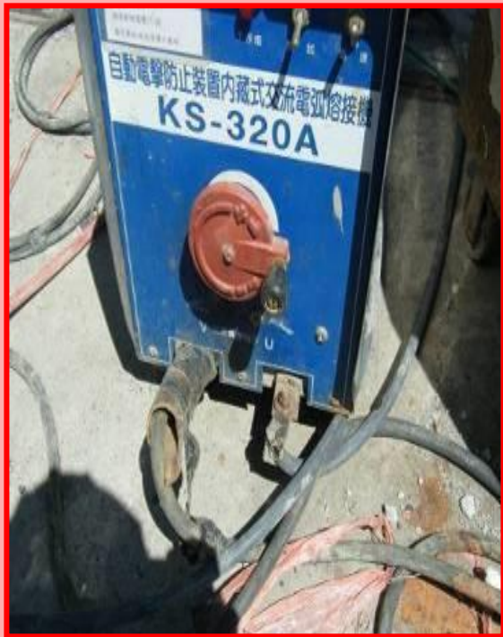
Before 接電端子裸露
